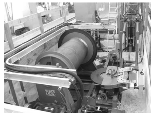
Fig. 9. Winch on the left and level wind in right foreground; cable runs around level-wind sheave to the second sheave at base of drill tower, barely visible in the background.
